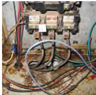
Corrosion leads to premature component failure
