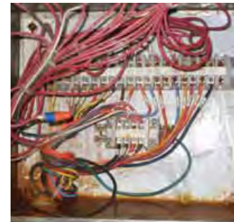
Water accumulation in electrical cabinet
