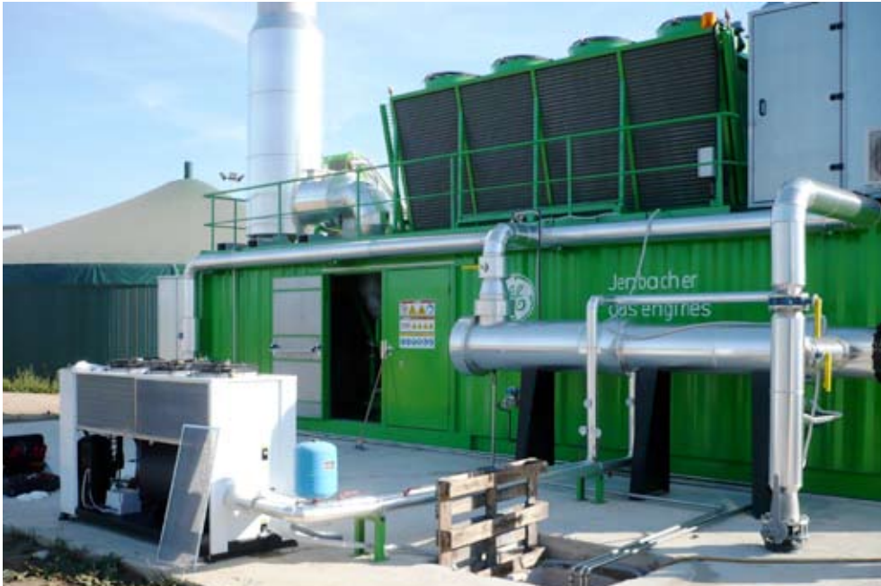
Cooling utilising Parker Hiross-Zander Solutions: WFS350 cooler SFH390 separator ICE150 Bio-energy Chiller
