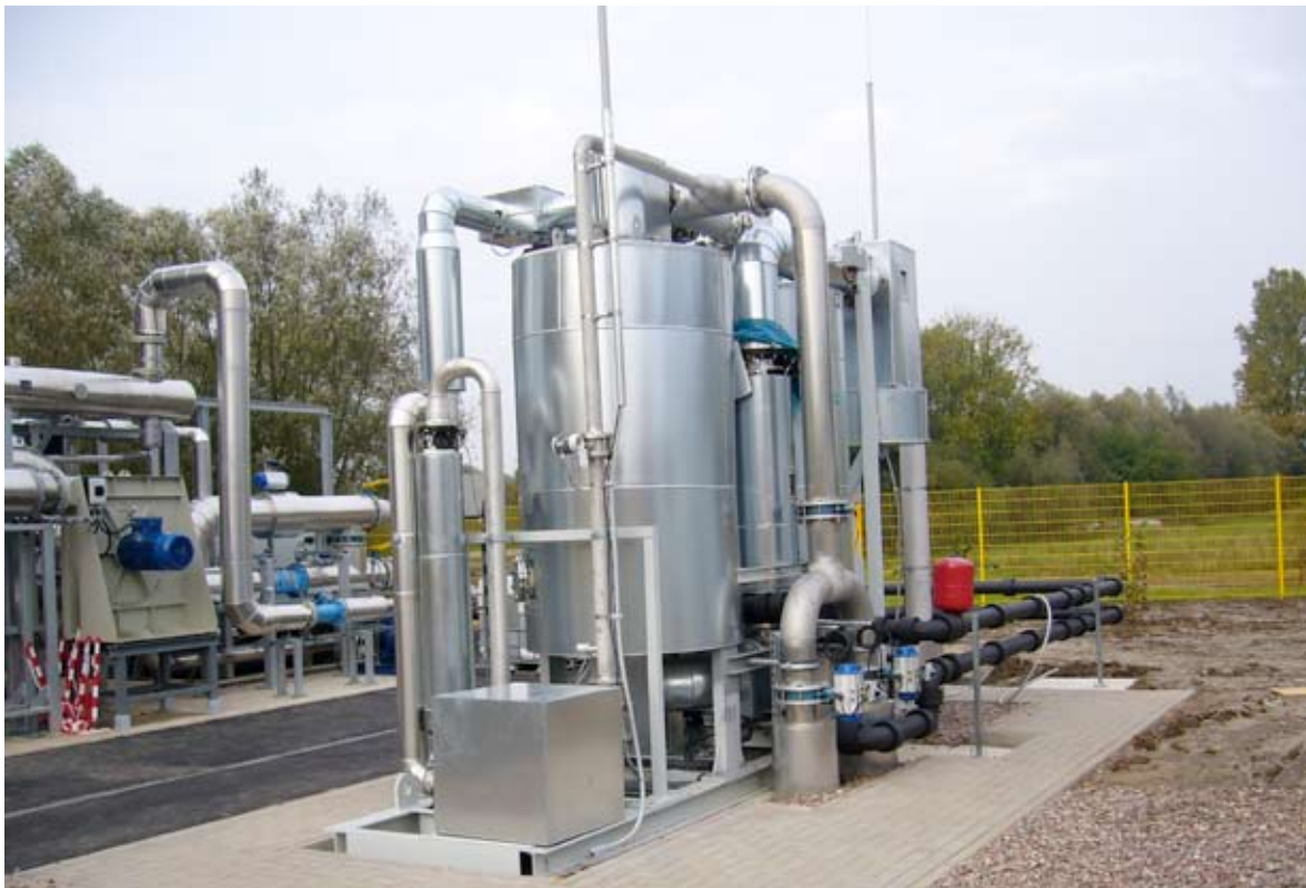
Type "W"-dryer with process gas regeneration. This principle represents a zero loss process, using methane as flash-gas
