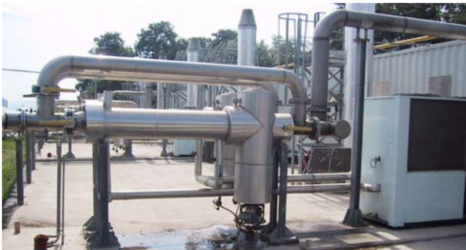
Cooling utilising Parker Hiross-Zander Solutions: WFS350 cooler SFH390 separator ICE150 Bio-energy Chiller
