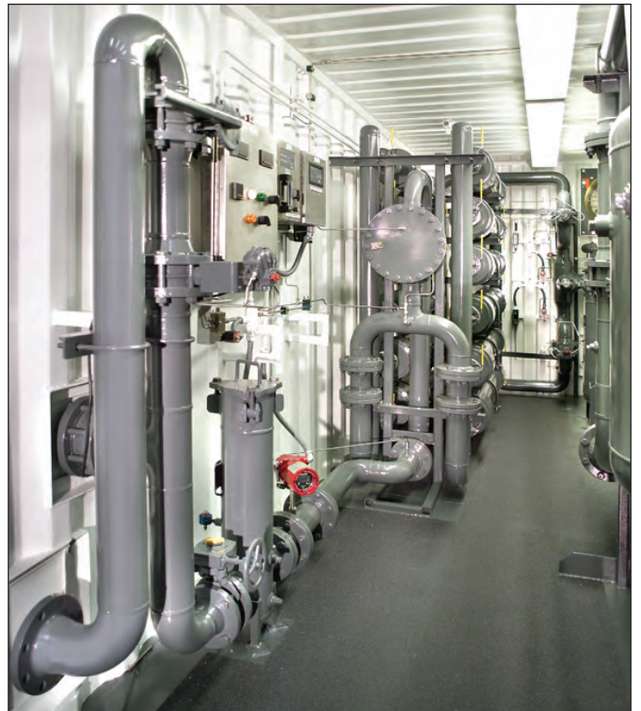
Interior View of Containerized System
